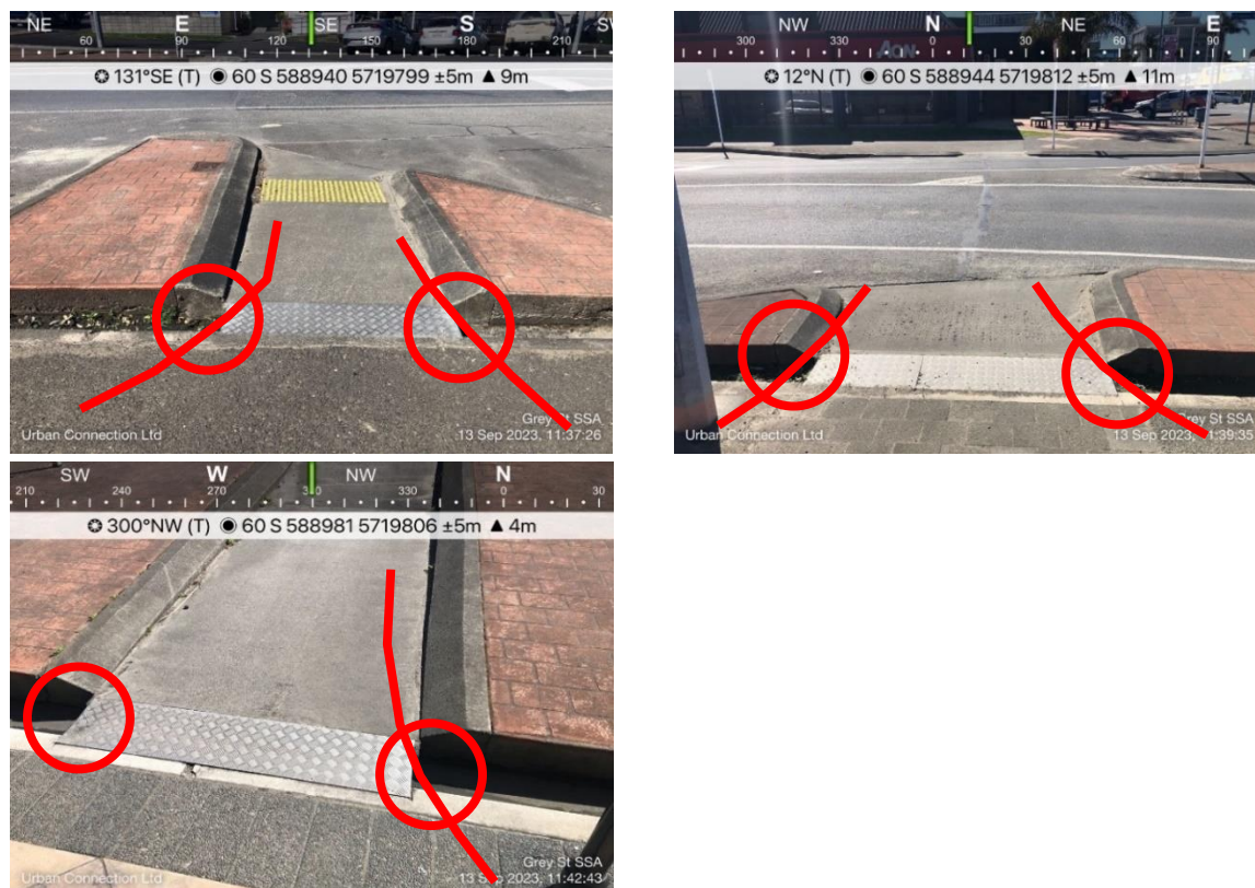
Figure 5.3-30 – Plate on the drain at crossings – tripping hazard
