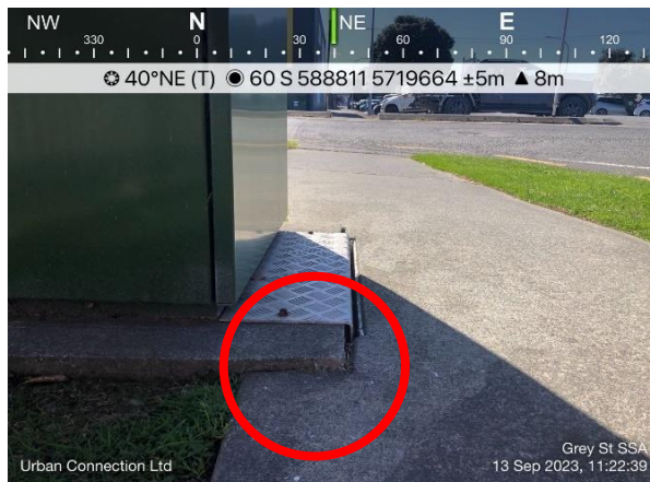
Figure 5.3-26 – Tripping hazard – lifted base of the high voltage box
