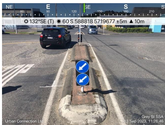
Figure 5.3-21 – Substandard pedestrian refuge on Kahutia Street West
