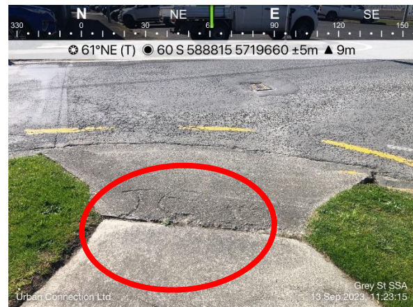
Figure 5.3-27 – Tripping hazard – lip in the ramp on Kahutia Street
