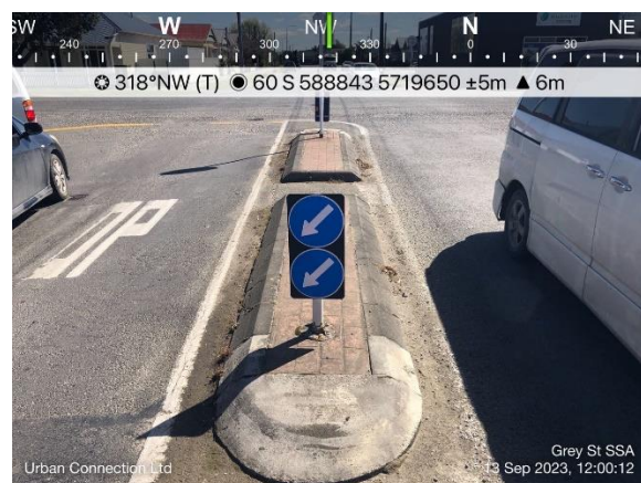
Figure 5.3-22 – Substandard pedestrian refuge on Kahutia Street East
