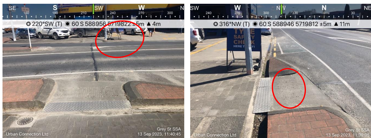
Figure 5.3-12 – Missing tactile pavers at crossing points across Childers Rd (west of Grey St)
