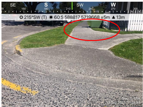
Figure 5.3-14 – Missing tactile pavers at crossing point across Kahutia Street (west of Grey St)
