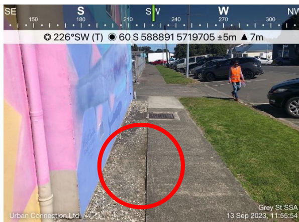
Figure 5.3-28 – Tripping hazard – level difference on the westbound footpath
